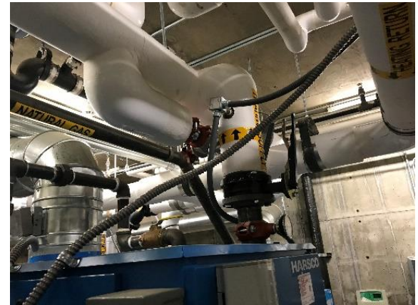
Boiler Pipe Loop
