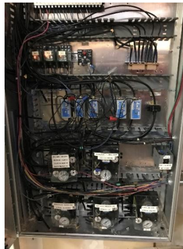
Pneumatic Control Panel
