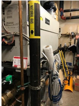
Old Draft Air Boilers
