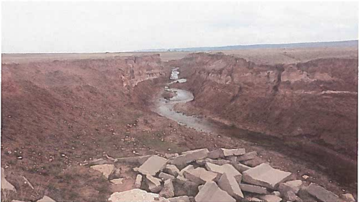
Photo. Looking north at section of Goforth Reservoir dam that was compromised in the early 1980's.
